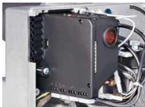
Control box fitted with ignition transformer
