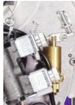
1 st stage air damper adjustment
