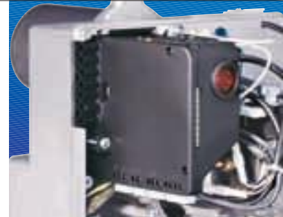
Control box fitted with ignition transformer
