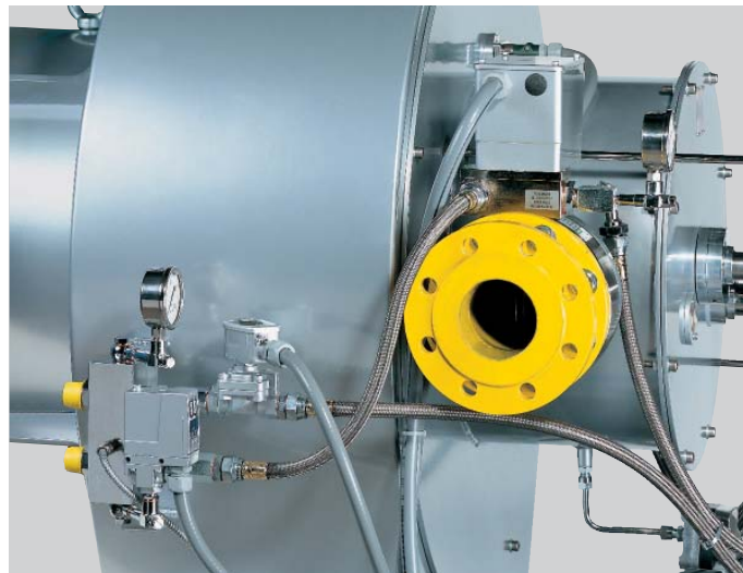
Example of oil and gas unit ER 9
